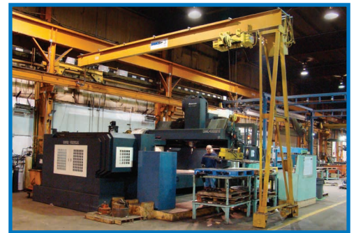
A 3-Ton Spanco Single Leg Gantry Crane with one end supported on the wall and one end traveling along the floor.
