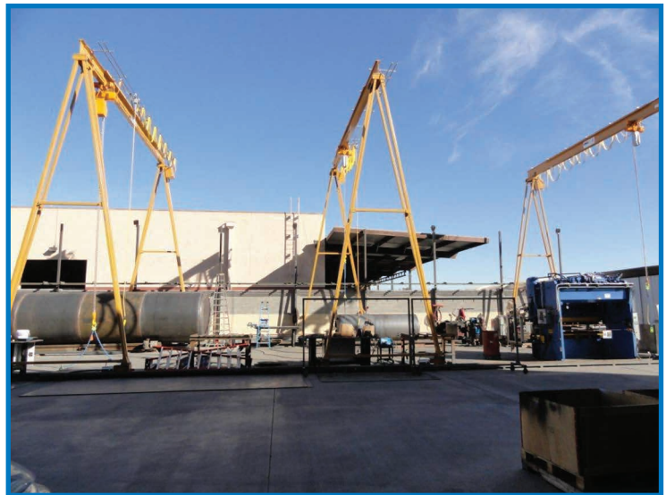
Three track-mounted PF Series Gantry Cranes mounted over rail cars for easy maintenance and repair. The track mount ensures smooth travel over a fixed route for increased productivity and ease-of-use.
