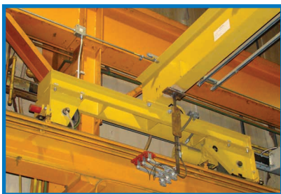
A Top-Running Single Leg Gantry Crane traveling along a ceiling-mounted runway.
