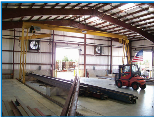
A 7.5-ton Motorized Spanco PF Gantry Crane used to move truckloads of long steel beams at a building material supply center
